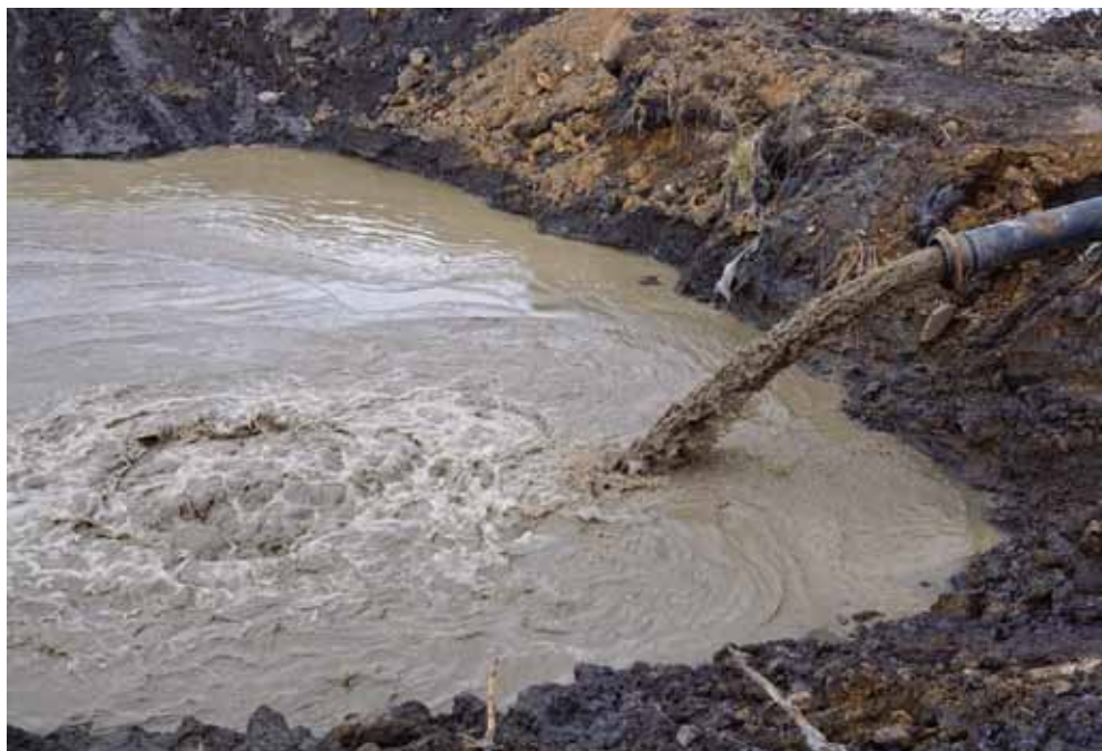
Ash and Water Discharge at Kingston Fossil Plant
